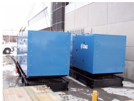
2 synchronized 910 kW SDMO Generators @ Purolator (see article below)
