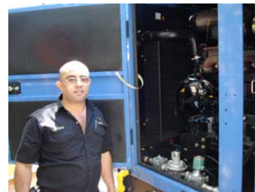
Elias Ayoub performing preventative maintenance on our on-site Bi-Fuel unit
